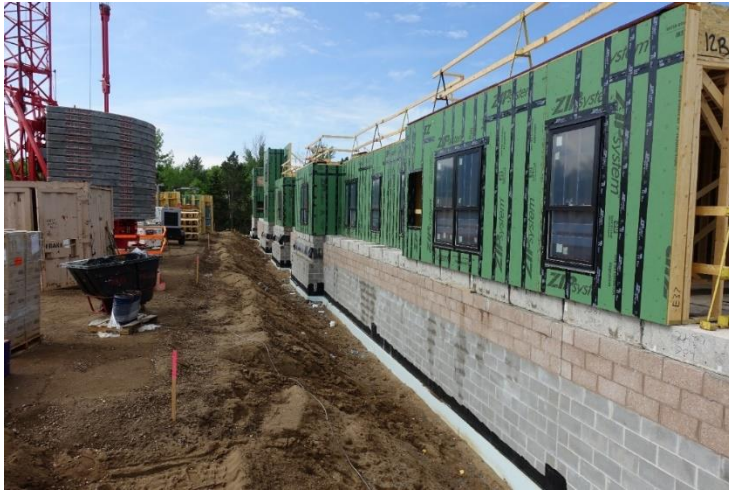
Panel wall joint at end of last wall panel installed at 1 st floor
