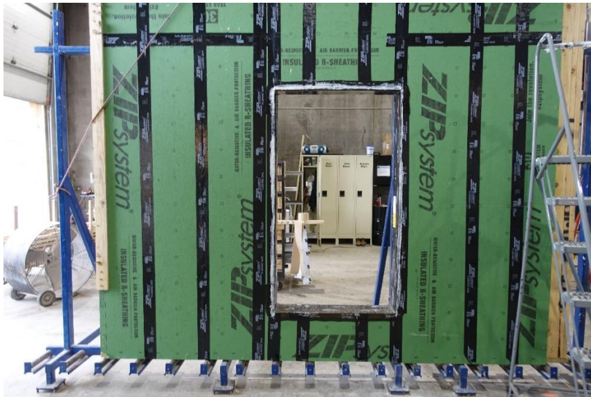
Wall panel at the factory ready for a window to be installed.
