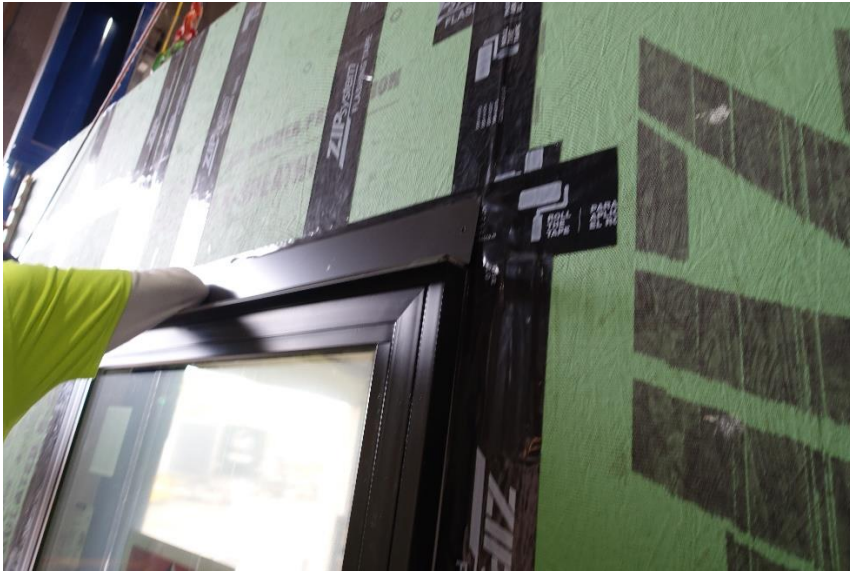
Installation of the top cap flashing on the window in the factory.
