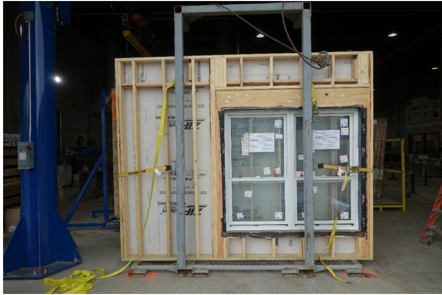
Wall panel at the factory with window installed. Note gray shipping frame.
