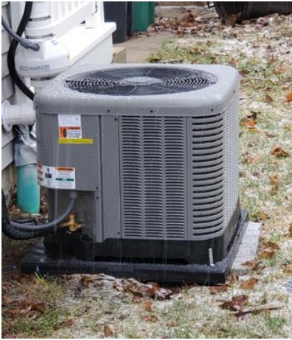
New Energy Efficient Air Conditioning Units
